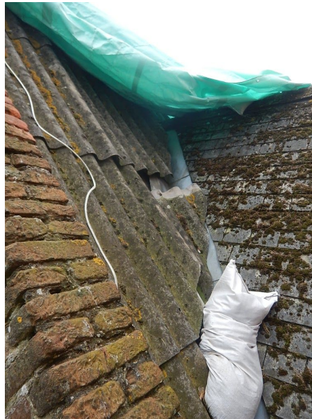
Lekken in de dakbedekking.
